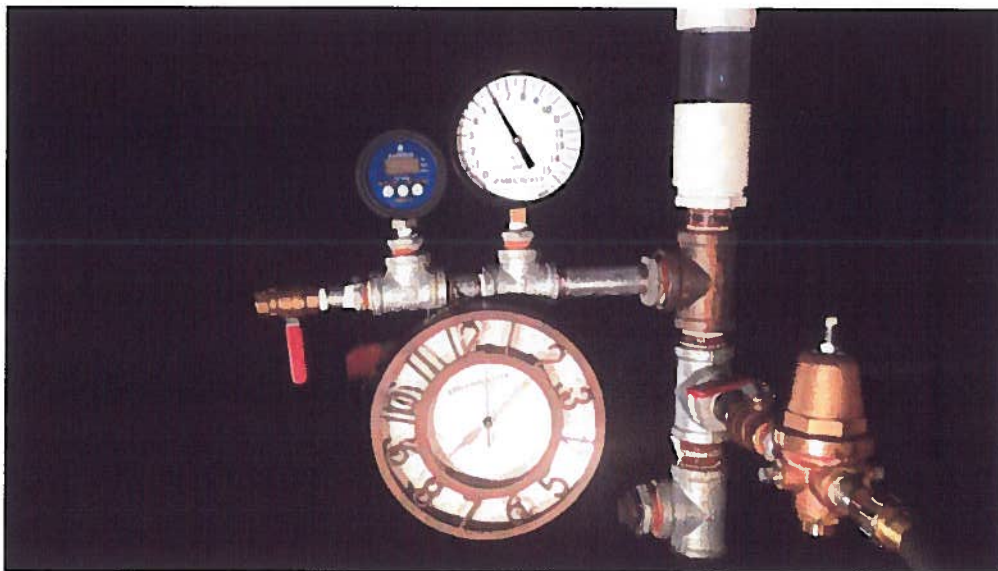
Water regulator, clock, pressure gauge and vertical water gauge connection
