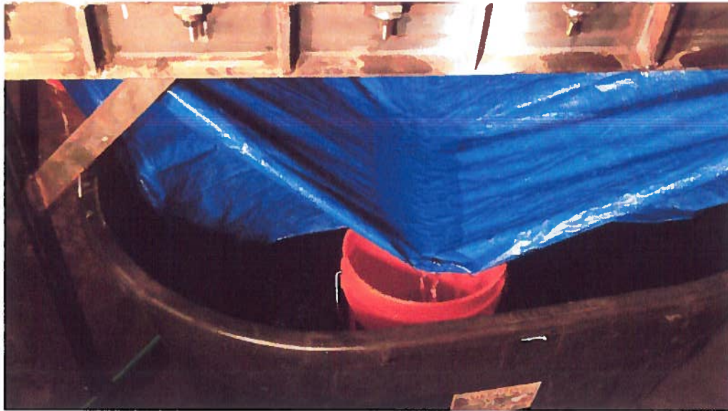
Water shown draining into the collection trough
